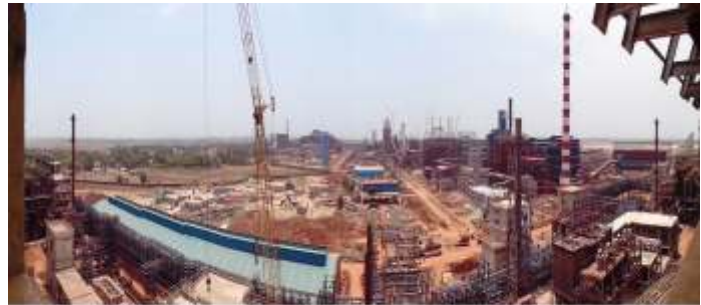
Panoramic view of upcoming Integrated Steel Plant of NMDC at Nagarnar under MECON's consultancy
