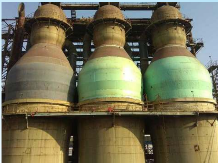
Conventional 3-section top fired stoves for 3x2500m 3 BF's converted into Yuxing 4-section top fired by cutting the top portion of the existing stove shell over 2000m 3 at Hebei Province which accounts for 2019, adoption rate of Yuxing top fired up to 84.6%.
