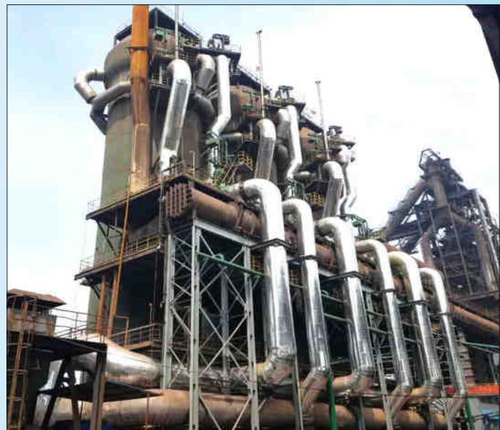
Internal combustion chamber stoves for 1497m3 BF at JianLong Steel converted into Yuxing top fired with a catenary dome
