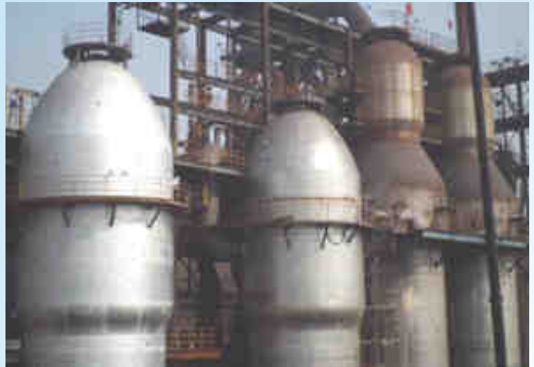
Conventional 3-section top fired transformed into Yuxing top fired with a catenary dome by cutting the top portion of the existing stove shell
