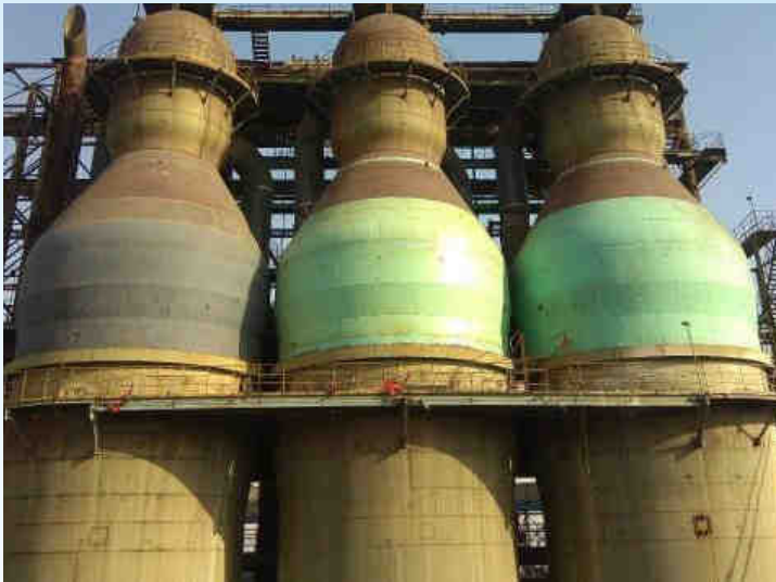
Conventional 3-section top fired stoves for 3x2500m3 BFs converted into Yuxing 4-section top fired by cutting the top portion of the existing stove shell over 2000m3 at Hebei Province which accounts for 2019, adoption rate of Yuxing top fired up to 84.6%.
